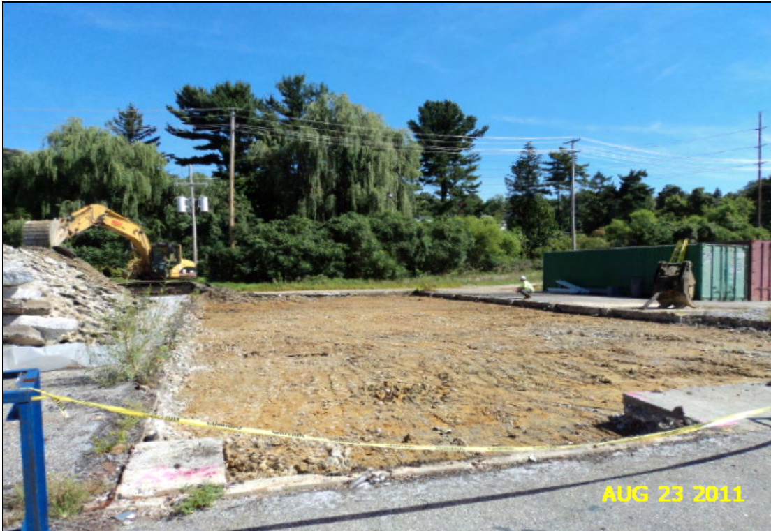
Photo 3: View looking north at Building 51 following demolition and removal of former hazardous waste storage pad and underlying gravel, and prior to confirmation sampling.
